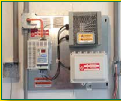
VFD Controls for variable speed operation
